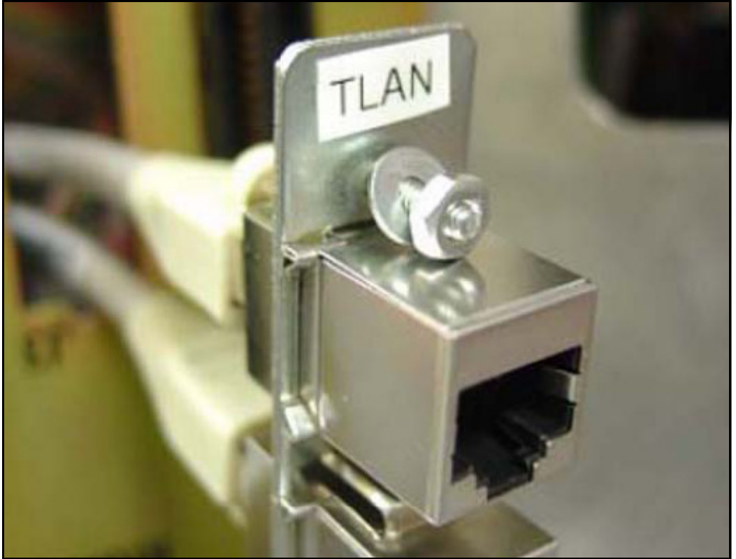
Figure 49 TLAN connection on Ethernet port coupler
