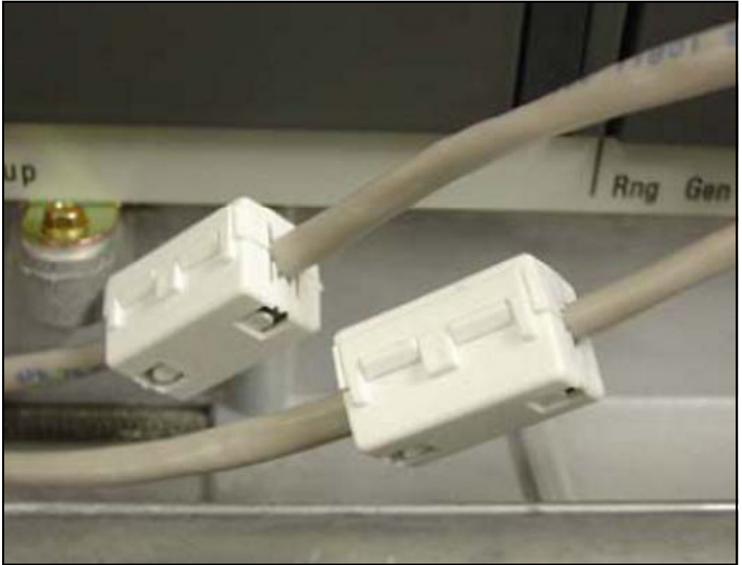
Figure 51 Attached Ethernet patch cable ferrite beads
