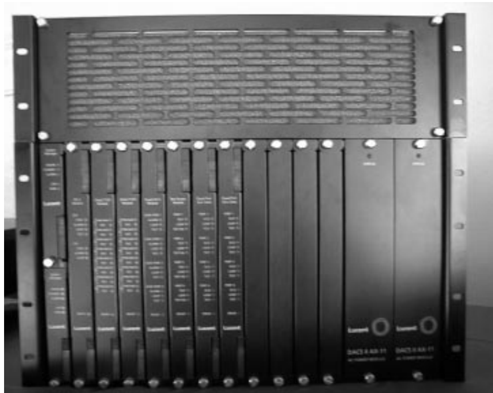
Figure 10-1. N+1 Protection Switch and DACS II AX 11
