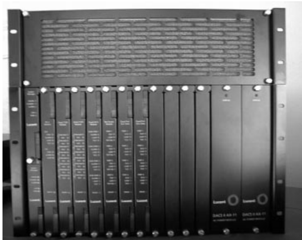
Figure 10-1. N+1 Protection Switch and DACS II AX 11
