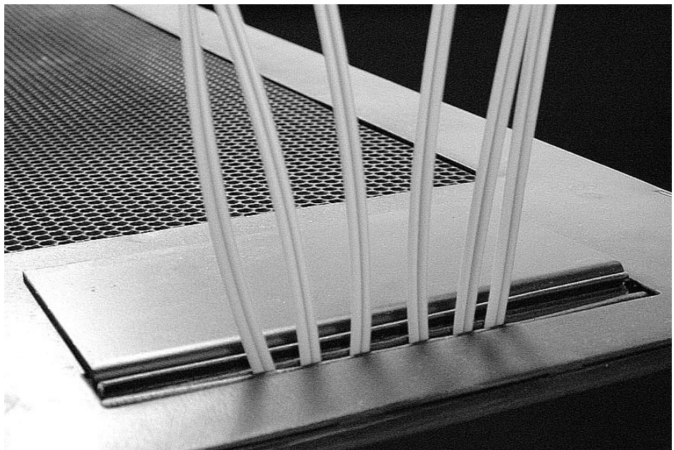
Figure 25. Positioning the Fibre Channel cable outside the frame
